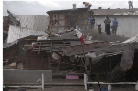
Roof collapsed under weight of the ash
